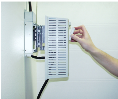
Installing the control panel
